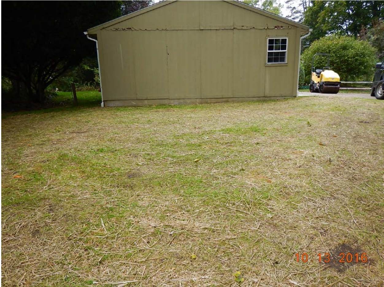
BACKFILLED SUBSIDENCE AREA
