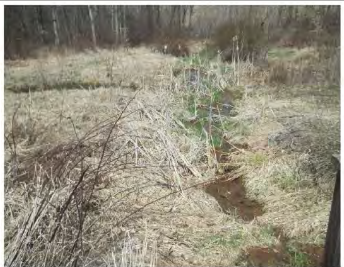
Outfall ditch from the southwest embankment of the flushing pond looking northwest
