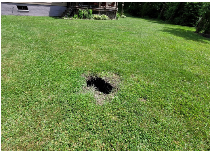
A close-up view of the growing subsidence in the yard, located directly above the collapsed top of the corrugated metal pipe
