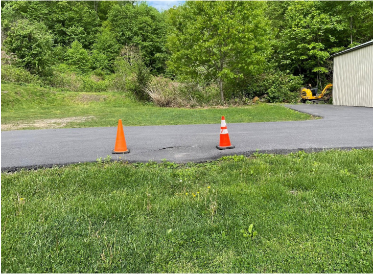
The collapsed corrugated metal pipe created a subsidence in the driveway and yard of the residence at 130 Sickler Hill Road
