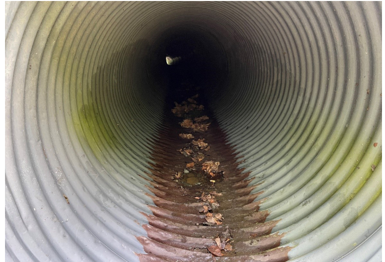
A view of the interior of the damaged 72" diameter corrugated metal pipe to be slip-lined with the 54" diameter snap-tite pipe
