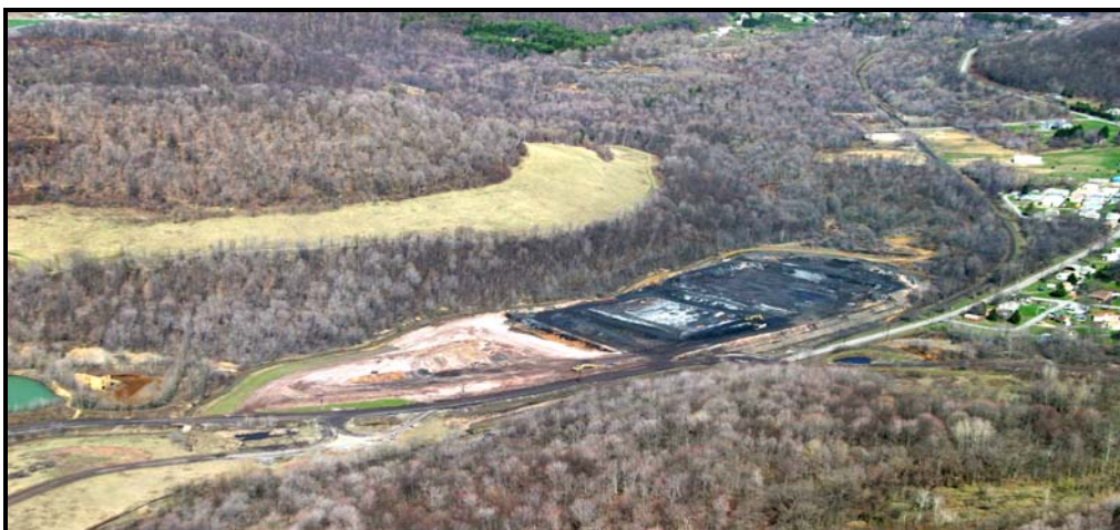
Barnes-Watkins refuse pile during reclamation; Phase 1, to the left, receiving FBC ash.
