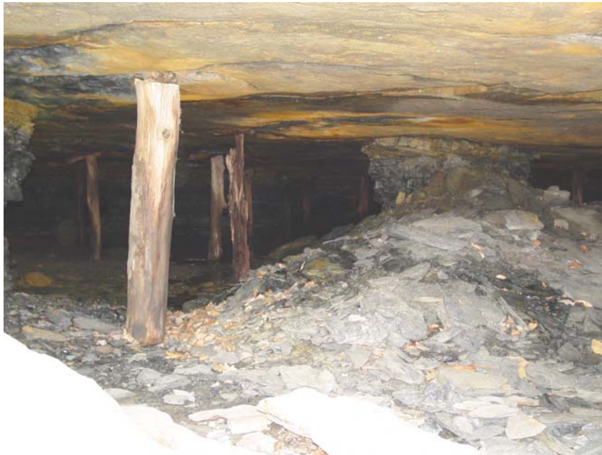
Close up view of mine opening AMLF No.17, the source of the water shown in the top photo.
