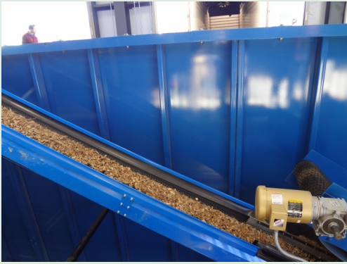
Biomass boiler feed conveyor
