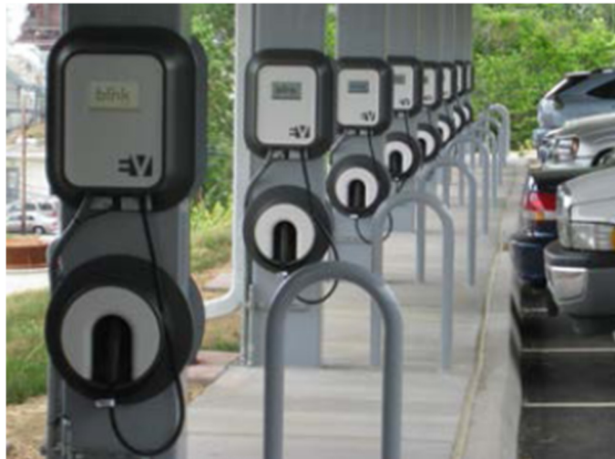
Figure 8 – Level II Fleet Charging Stations
