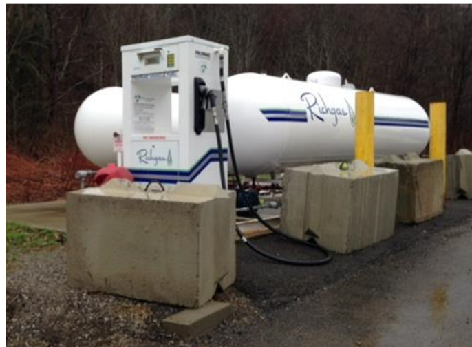
Figure 7 – Propane Fueling Station at Customer Site
