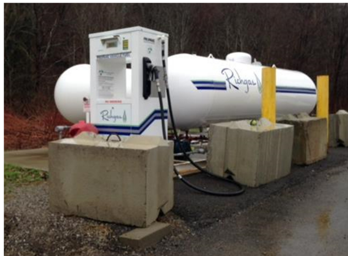
Figure 9 – Propane Fueling Station at Customer Site
