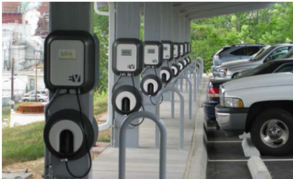
Figure 10 – Level II Fleet Charging Stations
