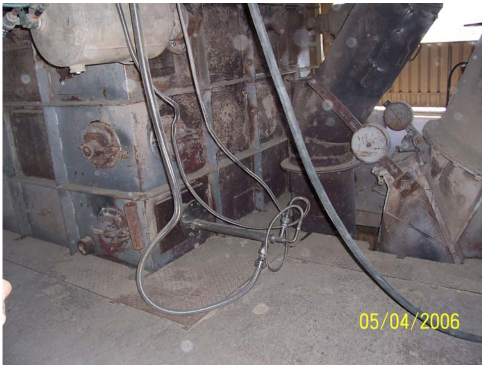
FIGURE 3 SNCR ammonia injections.
