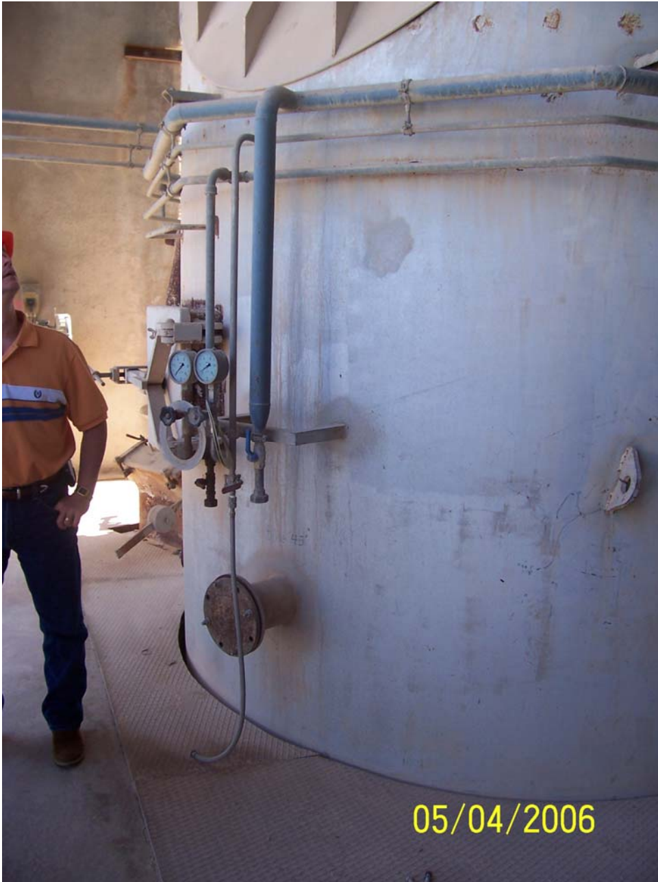
FIGURE 5 Disconnected SCR ammonia injection system
