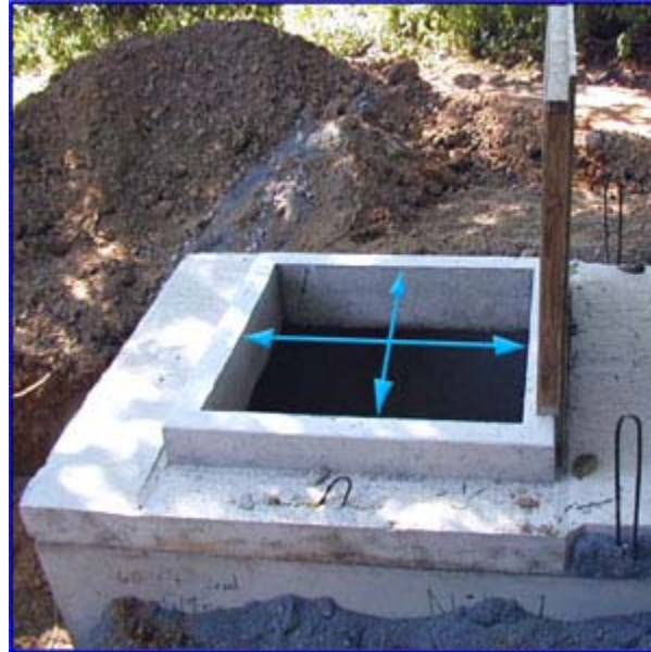
The photo shows one of the 36- by 36-inch access lids on the filter.
