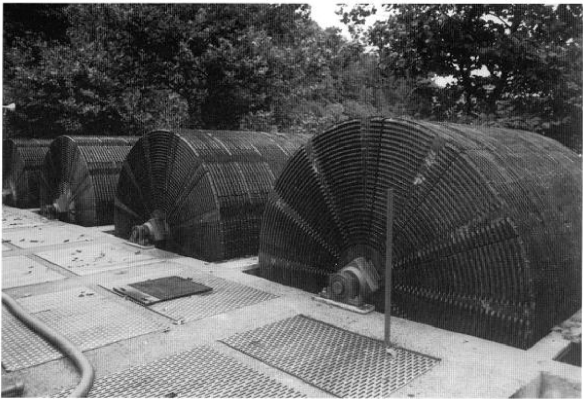
Figure 1.1 Rotating Biological Contactors 1
