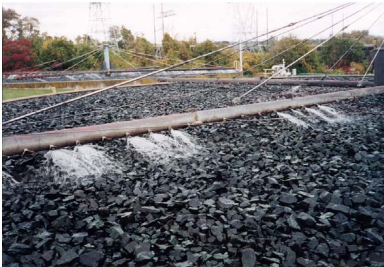
Figure 3.2 Tickling Filter with Clogged Nozzles
