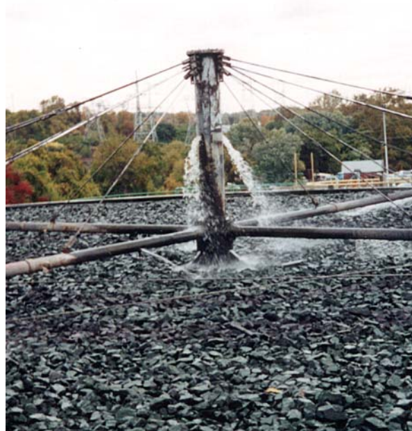
Figure 3.1 Tickling Filter with Leaking Seals
