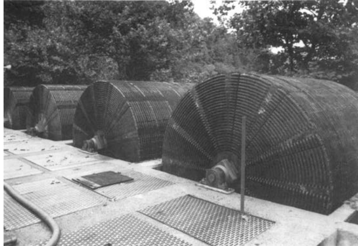
Figure 3.3 Rotating biological contactor 2
