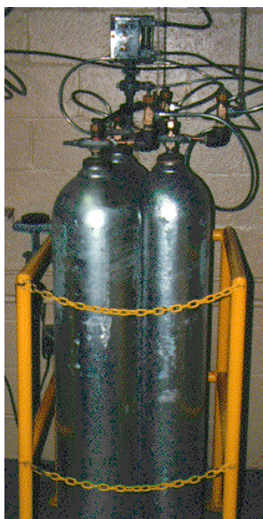
Figure 2.1 A 150 lb Chlorine Cylinder in Feed Position
