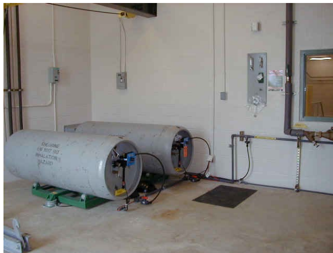
Figure 2.2 Ton Cylinders in Feed Position
