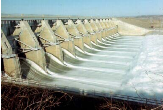
Gavins Point Dam Spillway. View of spillway 29,000 CFS Release. Missouri River. Yankton, SD.
