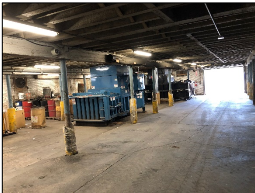
Baler Located in Lower Level
