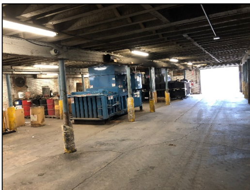
Baler Located in Lower Level
