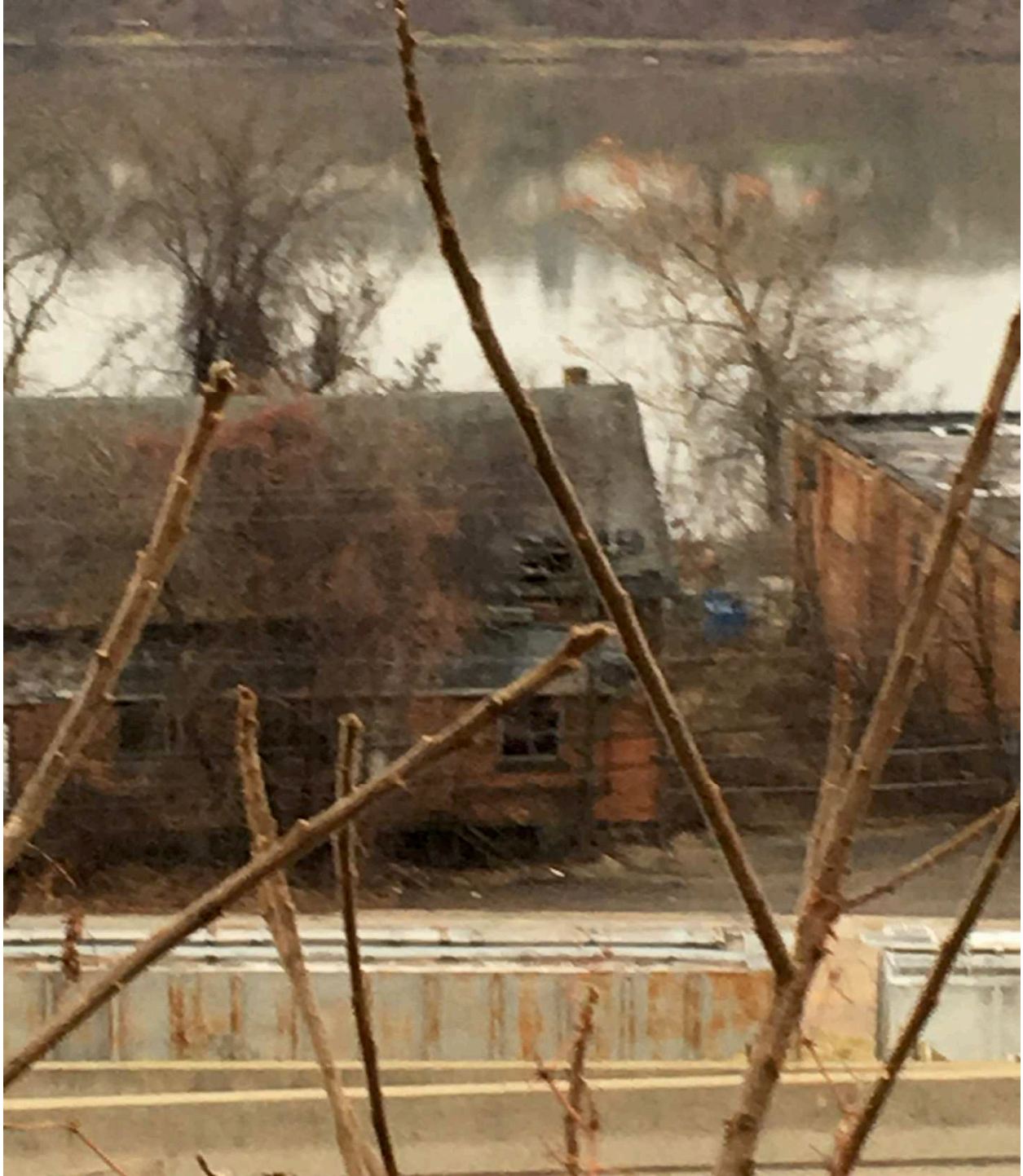
Hole in roof of Pool Doctor Building that contains several drums of waste
