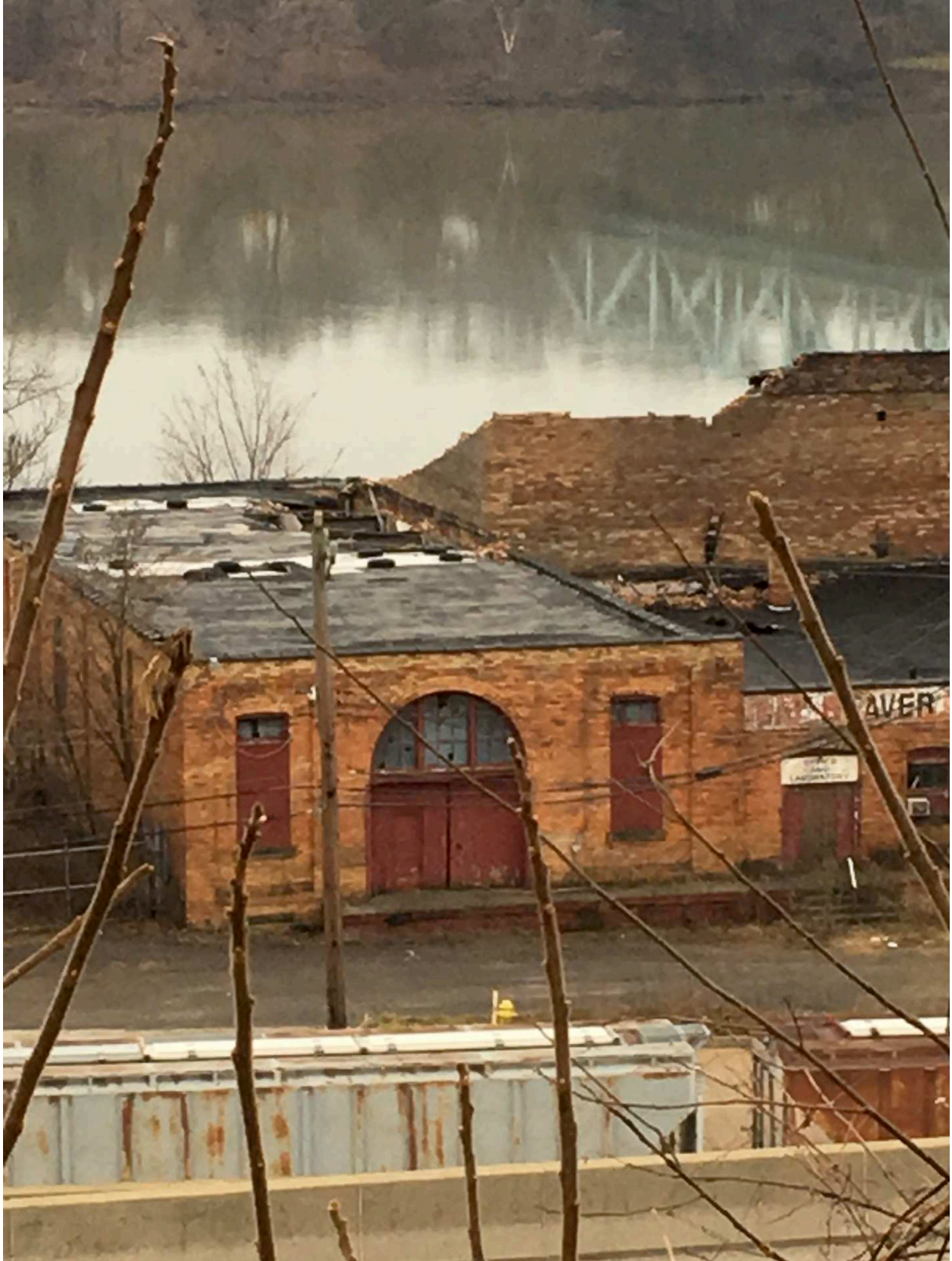
Collapsed roof of another Building that contains drums of waste
