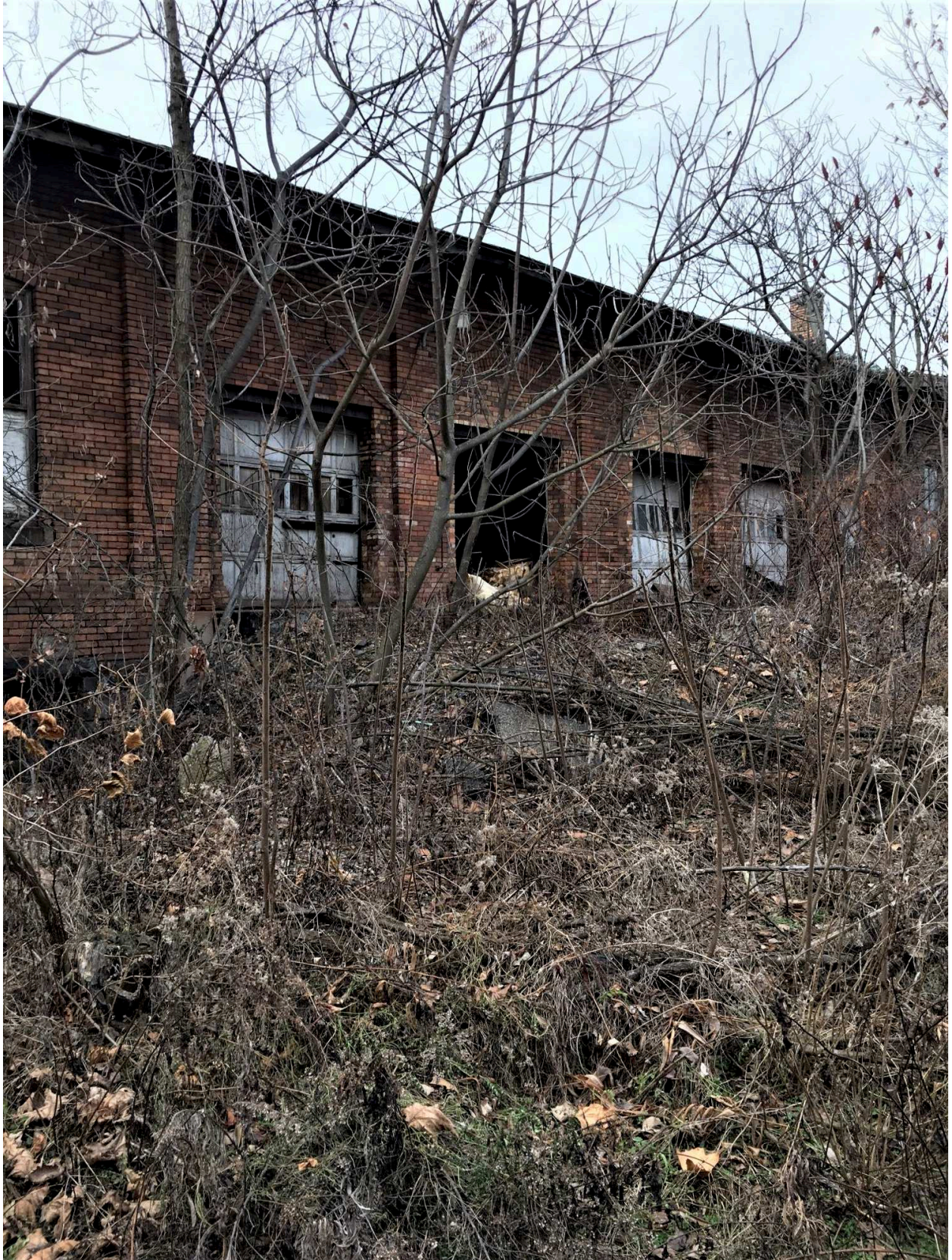
Missing door and drums sitting at the entrance. Strong odors are encountered at this photo spot.
