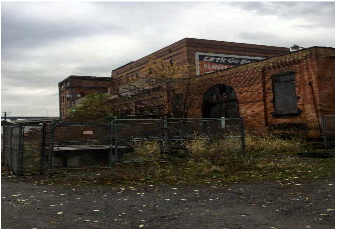
Laboratory part of Pool Doctor business, this area has a collapsed roof.
