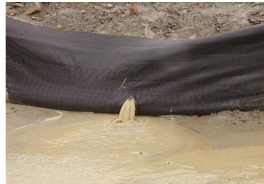
Failing silt fence
