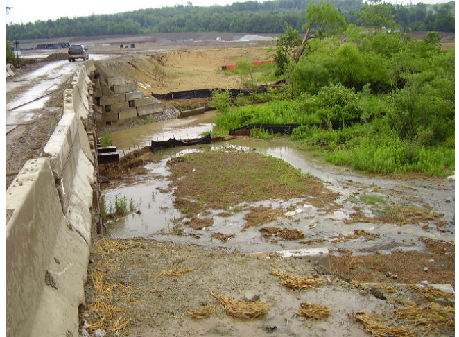
Erosion and Sedimentation / active development upstream of 6WC.
