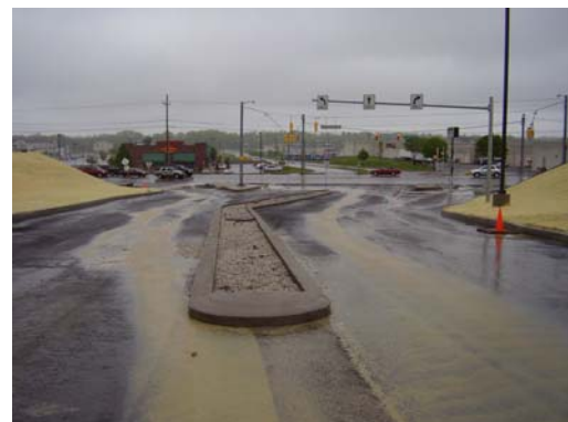
Stormwater runoff from an active development site along Interchange Road
