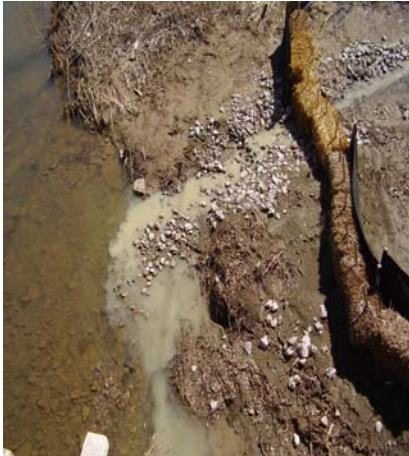
Stormwater Runoff from development upstream of 6WC
