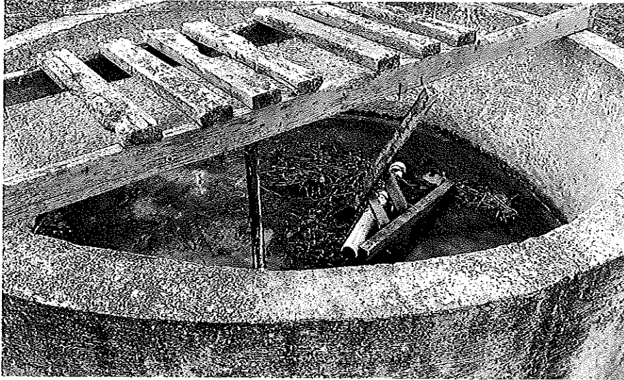
3/1/14 – Loss of water to developed spring after Emerald’s longwall mining
