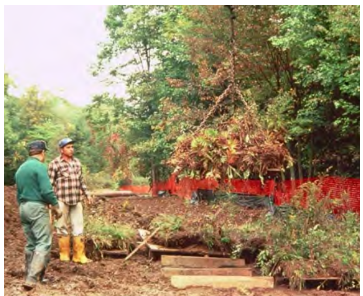
Stockpiling of forest soil and roots for later replacement over the pipeline trench, L. Sauer
