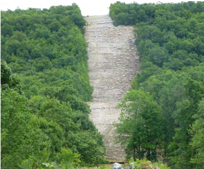
Attempted stabilization of a pipeline ROW on steep slopes, J. Zenes
