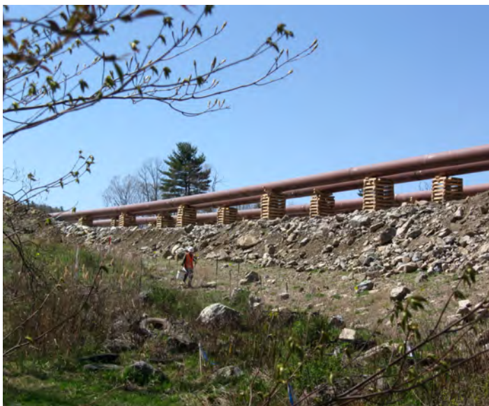
Pipe for the 325 Loop of Tennessee Gas Pipeline Co.'s 300 Line project in cradles in the New Jersey Highlands, J. Wagner
