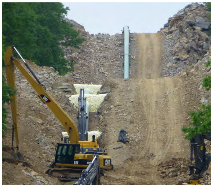
Key changes could reduce harms resulting from pipeline construction, M. van Rossum
