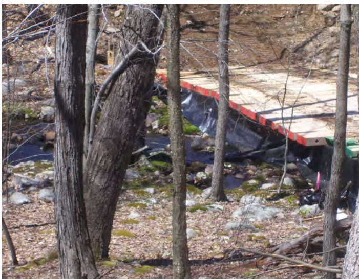
Tennessee Gas Pipeline Company's crossing of Shimers Brook, a trout stream in New Jersey, J. Zenes
