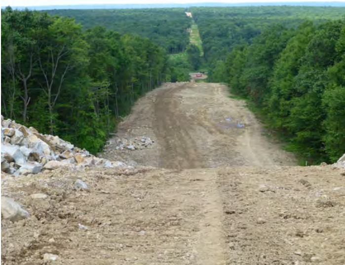
Pipeline cuts are invasive, damaging and permanent. Looking west from Kittatinny Ridge towards Pennsylvania, J. Zenos
