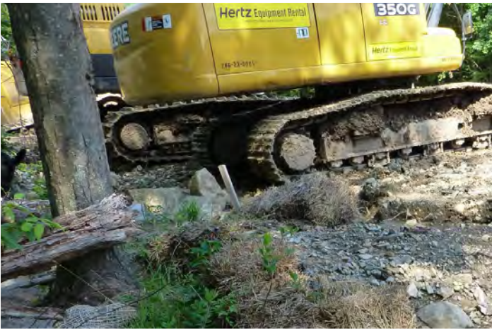
Pipeline construction practices can result in tree death even for trees outside the disturbance zone, J. Zenes
