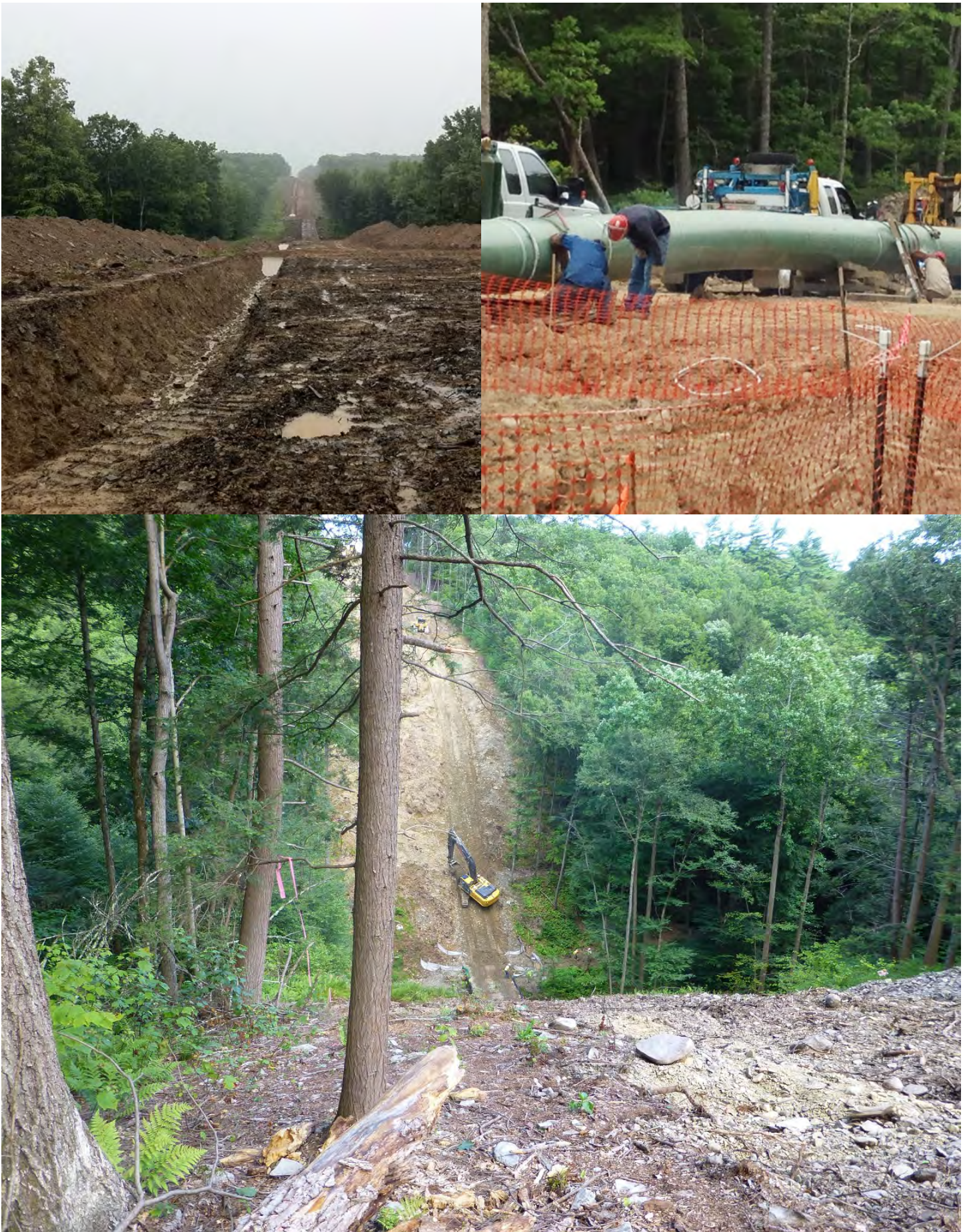
Clockwise from top left: Columbia Gas Company's pipeline ROW carving across Pike County, PA, F. Zerbe; Construction of the Tennessee Gas Pipeline Company's North East Upgrade project, F. Zerbe; Removing sediment from Cummins Creek, Pike County, PA, after a rain event, J. Zenes
