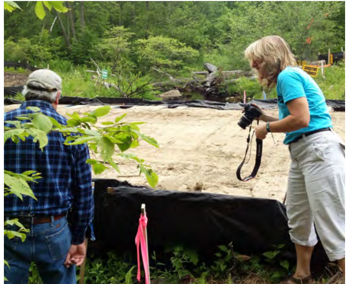
DRN staff monitoring a construction crossing of Big Flat Brook, a trout stream, in High Point State Park, New Jersey, F. Zerbe
