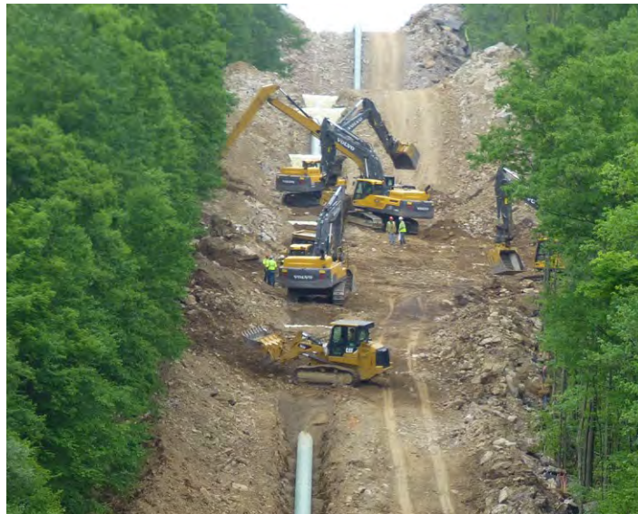
Heavy construction equipment backfilling a trench along a pipeline ROW, F. Zerbe
