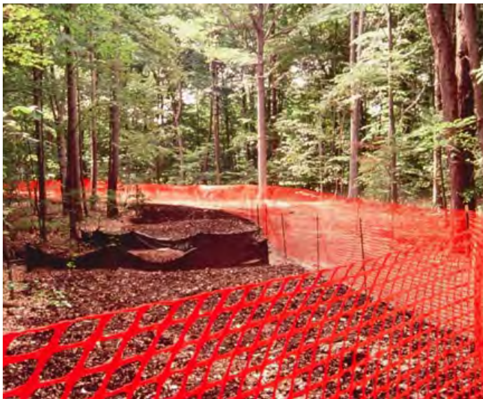
Pipeline ROW fenced immediately after construction to protect newly replaced forest sods and to define long-term access routes, L. Sauer
