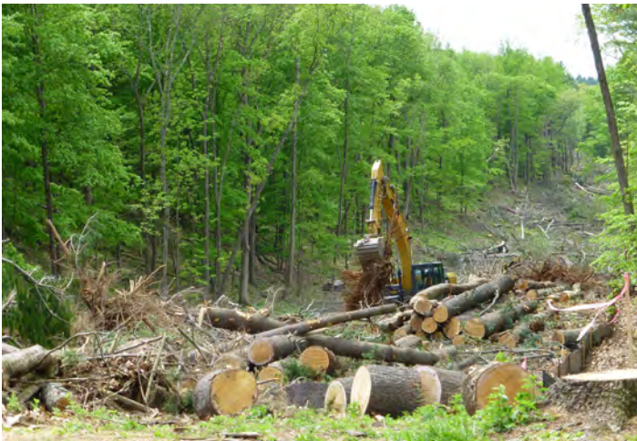
Clearing forested wetlands in Montague, New Jersey, in advance of pipeline construction, J. Zenes
