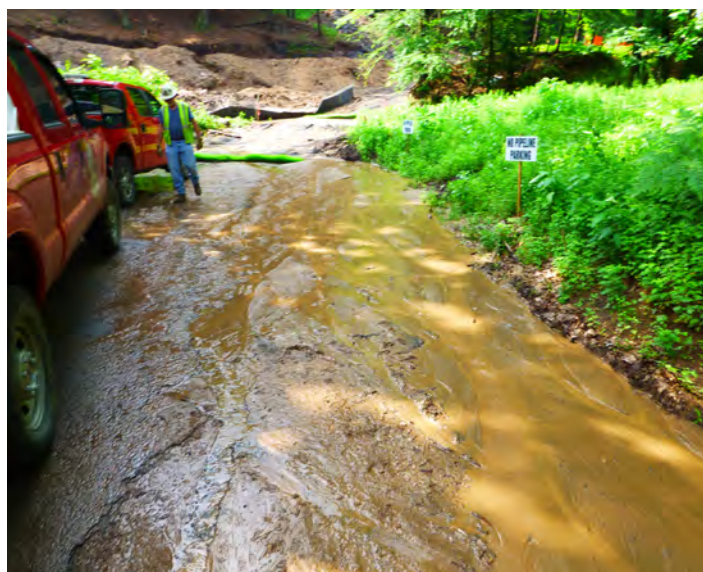
Failure of erosion controls at pipeline construction site Mountain Road Montague, New Jersey, J. Zenes
