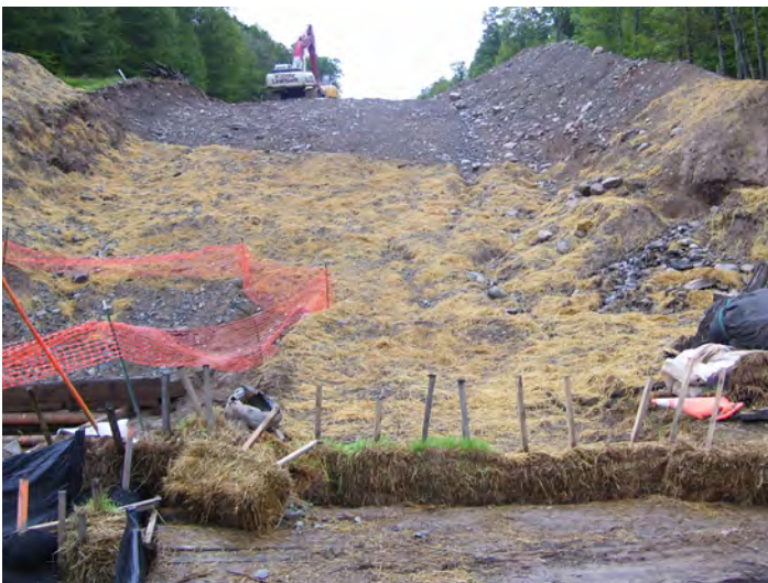
An overly wide pipeline ROW, M. van Rossum
