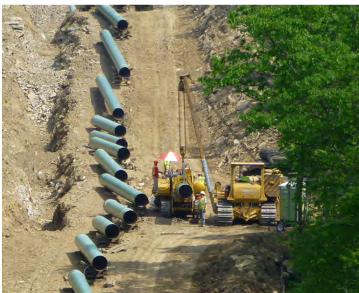
A side boom preparing to lower pipe into a trench, J. Zenes
