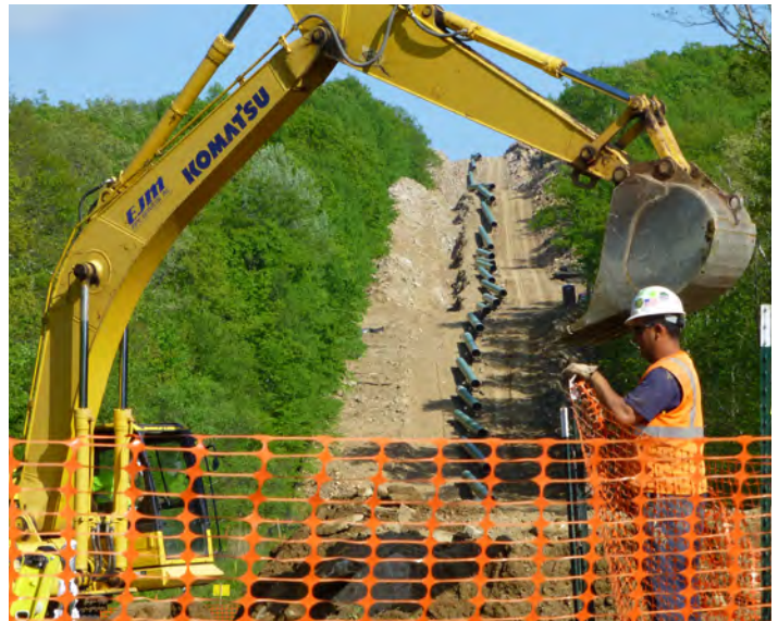
Pipeline ROW work on Kittatinny Ridge in New Jersey's High Point State Park, M. van Rossum
