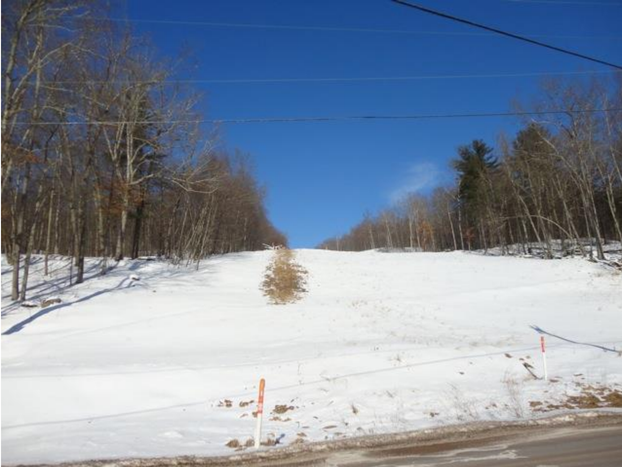
Winter snow melt over 30 inch buried pipeline, February 18, 2015. Photo by J. Zenes
