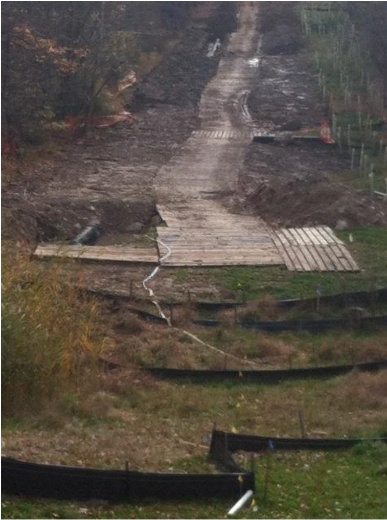
Maintenance work conducted by TGP on the old 24 inch line in the Fall, 2014. Photo by J. Zenes
