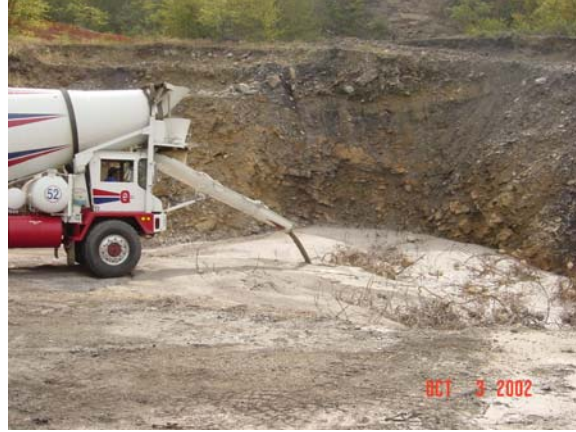
6.14(b). Grout added. Notice the mixer is driving on previously poured grout.
