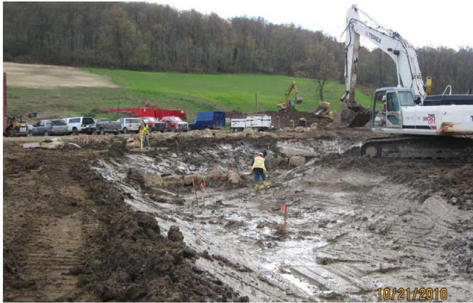
Figure VII-16. Placement of alluvial amendment liner into stream channel in E18 panel of Crafts Creek (Photo from PADEP files).
