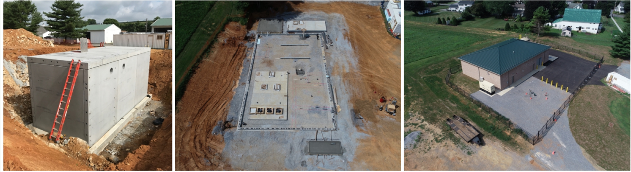
Water Treatment Plant (Left to Right) Installation of Clearwater Tank, Foundation and Floorplan, Completed construction
