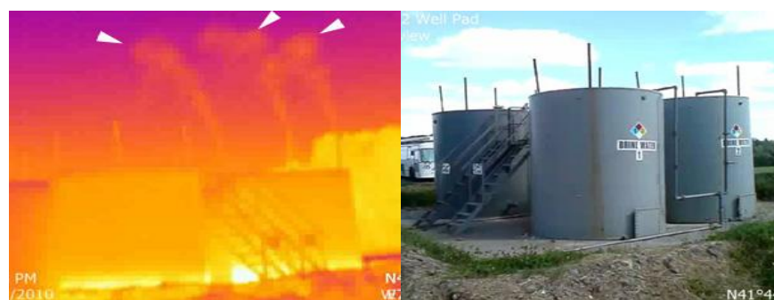
Figure 2 - Image of Natural Gas Condensate/Brine Tanks using Infrared Gas Detection – The left image shows the emissions of gas from the tank vents (denoted by the three arrows) using the gas detection camera. The right image was taken at about the same time with the same camera in normal photography mode, although from a slightly different angle for lighting purposes. Source: PA DEP
